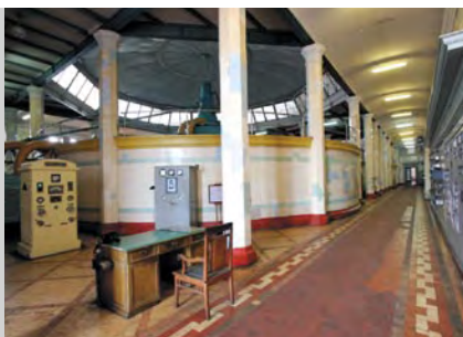
Inside Uglich hydro power station, Russia.
