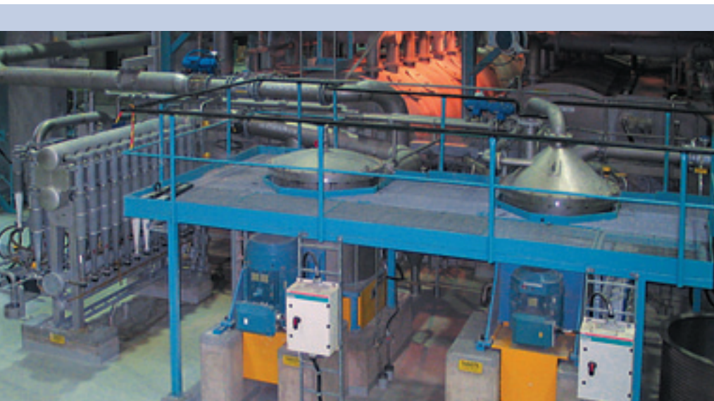
Blick in die Recycled Fiber-Anlage.
